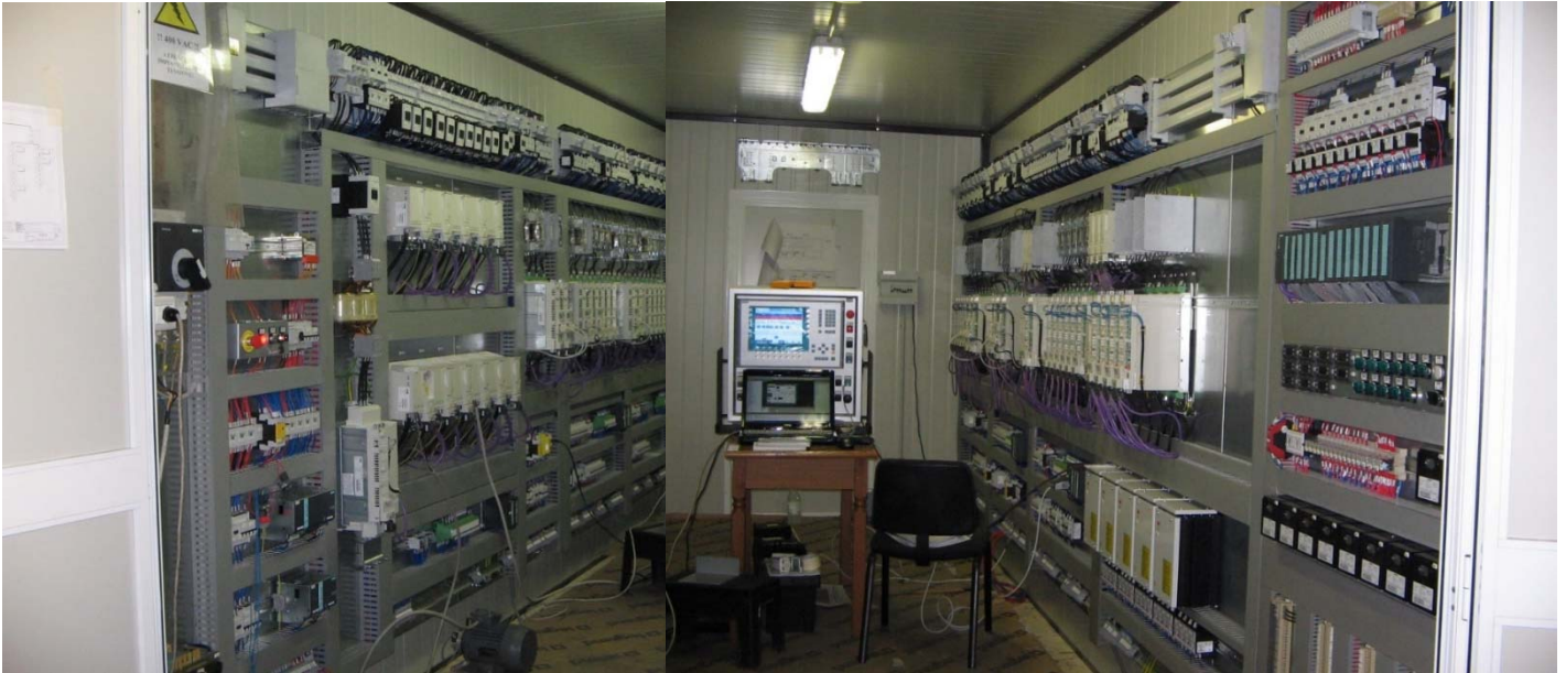
➤ Electrical Board supplied pre-assembled in Container
