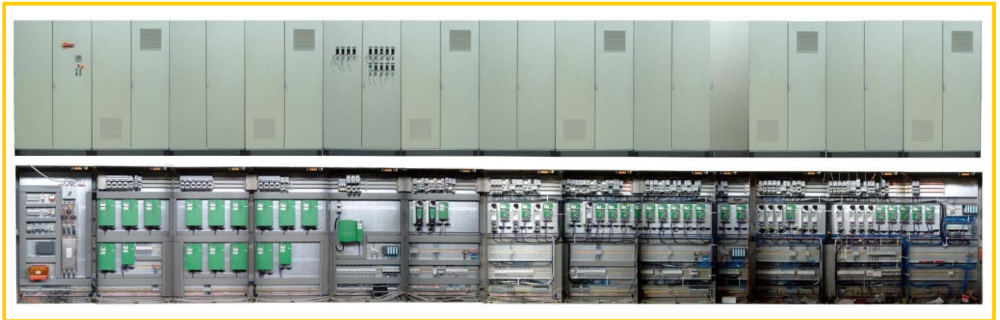
➤ Standard Electrical Board
